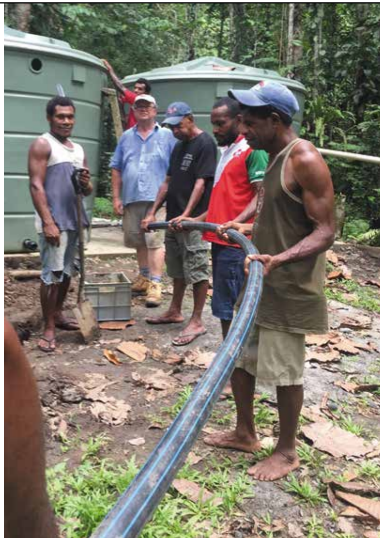
David Chambers about to connect the college water supply to the new 10,000 litre tanks, assisted by a number of the college students
