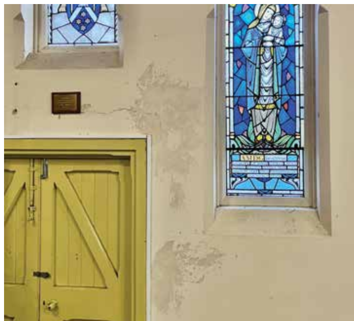
Damage to a section of the wall in the heritage church
